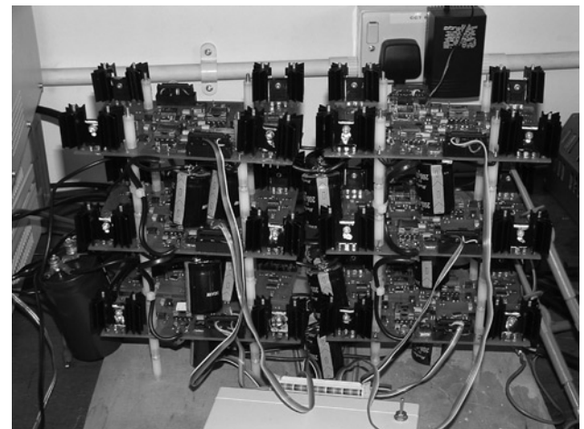
Fig. 8 Experimental four-cell five-level flying-capacitor inverter assembly
